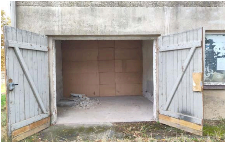
Garage [ Dorfstr 53 Gutshof] Sound installation | Bevand | Rao |
